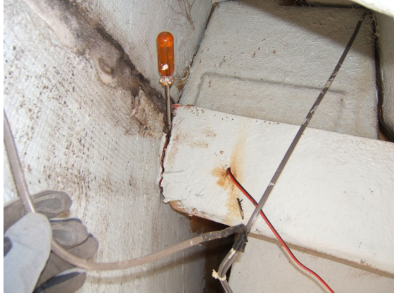
Main beam port side
